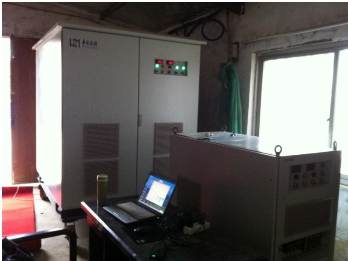
Fig.9 DC power source for large scale application
