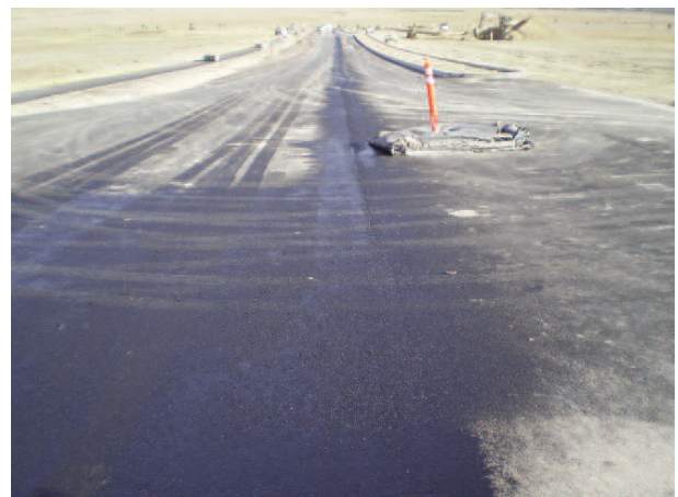
Final lift of asphalt will be placed before open to final service.
