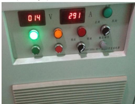
Fig.5 Automatic DC power source
