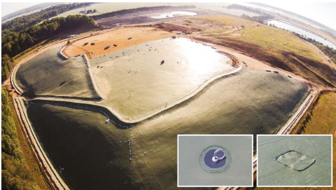
Aerial view of the completed project. Inset photos show the anchor once installed and after placement of the HDPE patch to seal the geomembrane.
