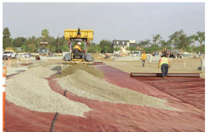
Placing Mirafi® RS380i over native soil and applying base material over RS380i
