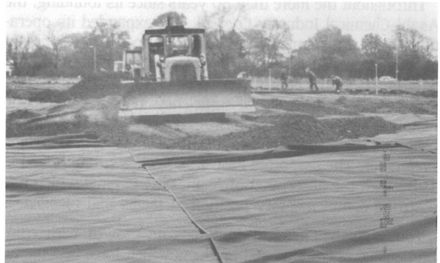
Lotrak 1 - Lotrak 35/30 used in separator and reinforcement application. A17 Long Sutton Bypass, England.
