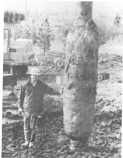
Fully automatic piling system "City Guy" for use in confined inner-city areas. Photo shows expanded pile base formed using a geotextile (see text).
