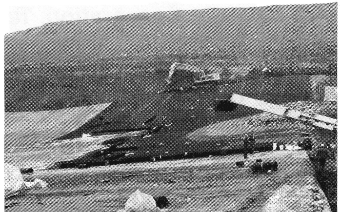
Protection of the synthetic lining in the Odenwald waste tip using geotextile/bentonite mat.
