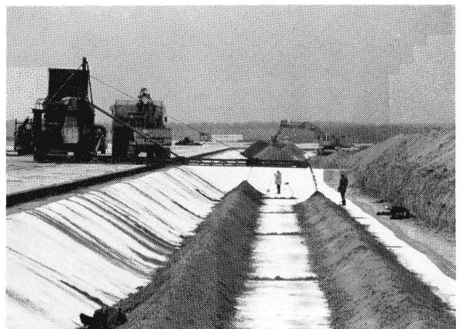
Lining of the ASG system with geotextile/bentonite mat liner at the Munich II Airport
