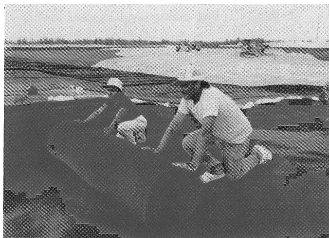
Landfill project in West Palm Beach Florida using Gundle Lining Systems products
