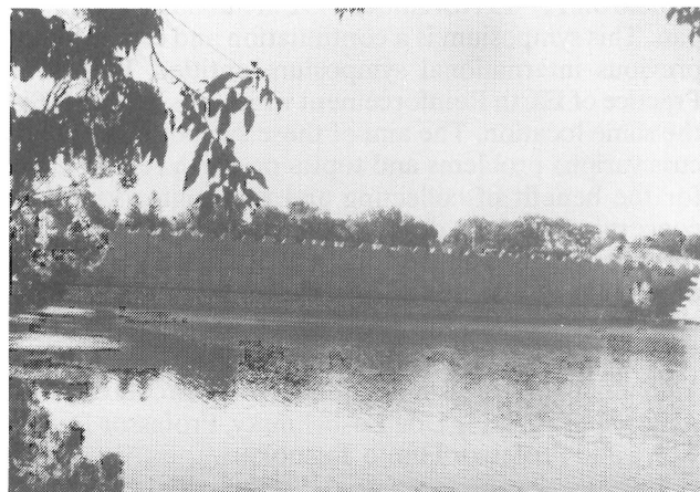
11m high Reinforced Earth wall placed over stabilized base at Route 16 project (just prior to completion)
