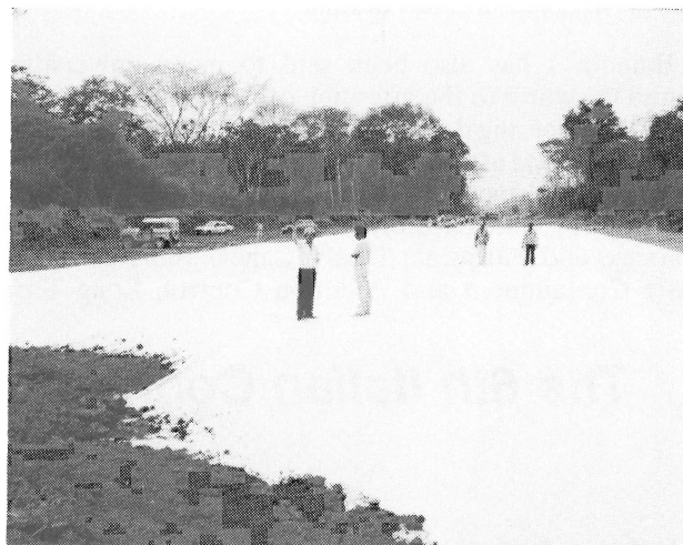
Construction of the Magdalena Medio road near Barrancabermeja in Colombia using 1.400 T PAVCO woven geotextiles.
