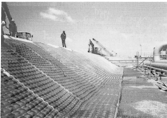
TACOM VSL MAT – Fabric Formwork Concrete Mats for berm slope protection of a oil retention pond in Iraq
