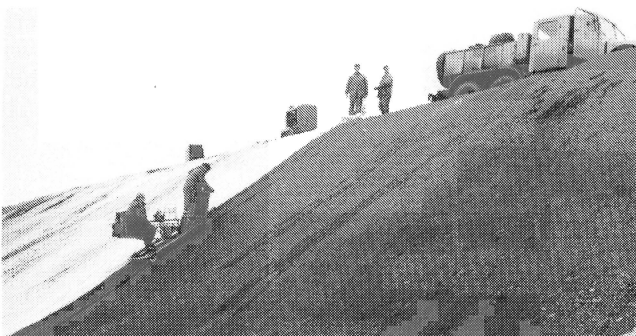
Geotextile filtration layer panels being sewn at the site of a mud retention pond
