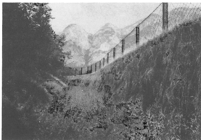
Polyester geogrid-reinforced embankment for protection against rock falls.
