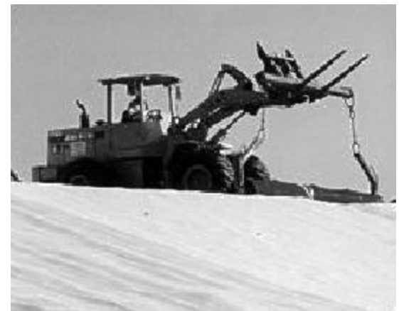
Bentomat ST and Claymax 200R GCLs used for the Mt. Airy, North Carolina, USA landfill.
