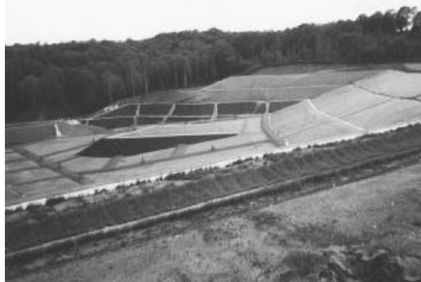
Installed geomembrane from a landfill project on Hokkaido, Island, in northern Japan.
