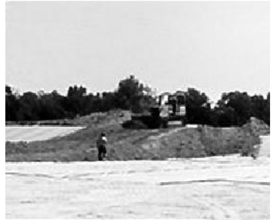
Bentomat CL and Claymax CL GCL liners used for City of Pangburn, Arizona, USA sewage pond construction.
