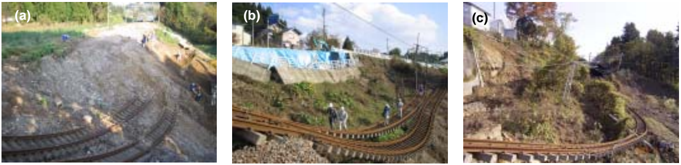
Figure 1. Three severely damaged embankments between Ojiya and Kawaguchi on the Jo-etsu railway line: (a) Site 1; (b) Site 2, compound failure of embankments on Highway No. 17 and the Jo-etsu railway line; and (c) Site 3, failure adjacent to a railway tunnel (7 November 2004, photo taken by F. Tatsuoka).
