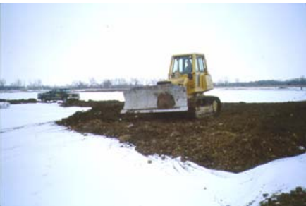
Figure 4. (a) Challenges during construction on extremely soft ground, and (b) capping of sludges using geotextile and wood chip-soil mixture.
