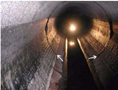
Failure of circumferential weld in sewer tunnel liner (PVC).
