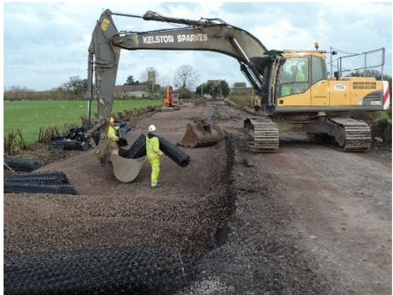
Stabilised access provided by a Tensar Mechanically Stabilised Layer which enabled construction operations to proceed quickly
